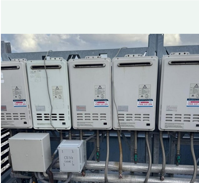
HOT WATER BANK
